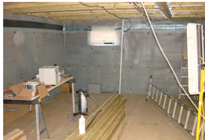
The basement was waterproofed using Platon P5 membrane on the wall and deeper studded Platon P20 membrane on the floor.
