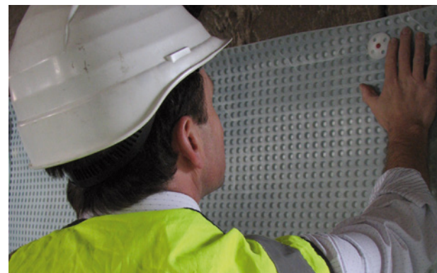
Cobb plugs were used to fasten the membrane in place of normal brick plugs
