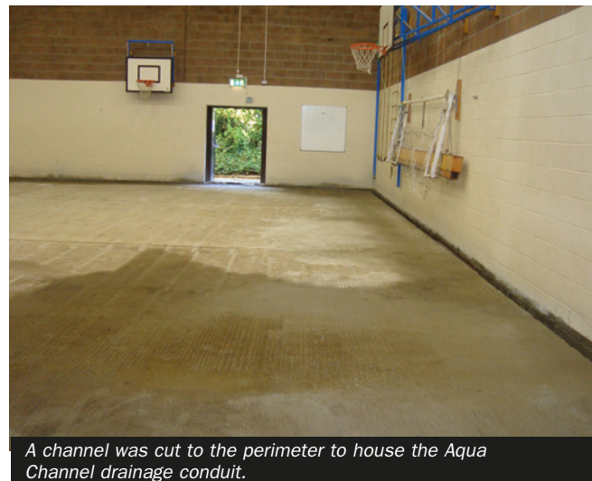
The failed system resulted in severe water ingress at wall/floor and floor/floor junctions.
